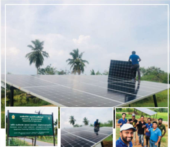
Agunakolapelessa Solar Water Pumping Project
